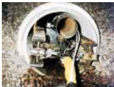
Clogged duct 600 mm.
